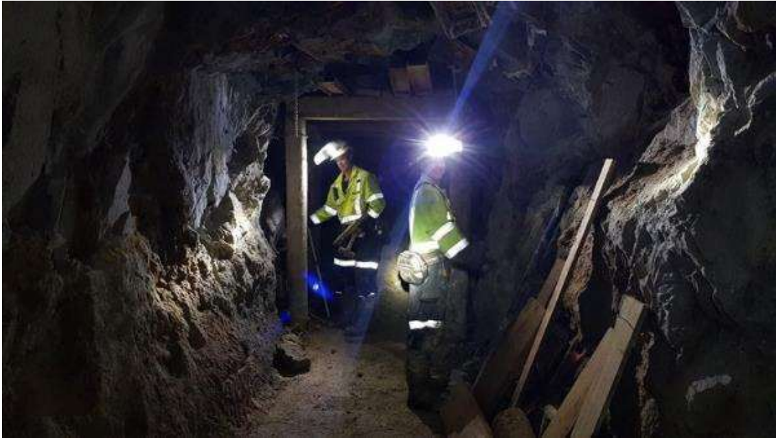
Figure 6 - Timber sets being constructed to reinforce the brow at the entrance to the Dubbo Rise
