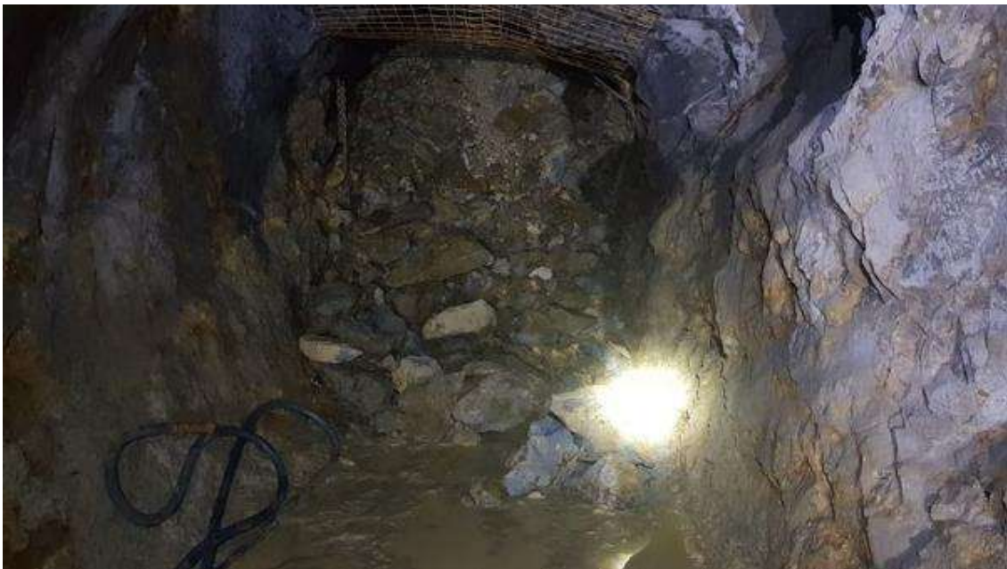
Figure 3 - the brow below the Dubbo Rise showing large material dislodged from the rise hangingwall.
